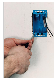
Secure Box in Wall
